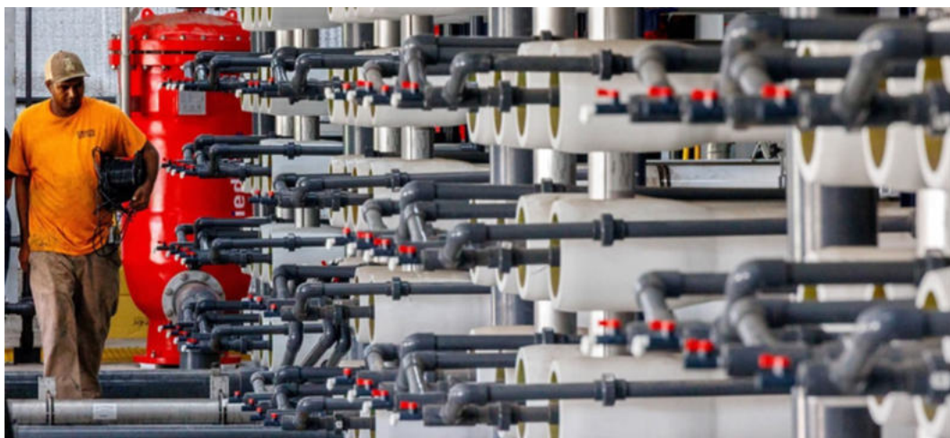
▲ Figure 2-33 St. Kitts and Nevis Smart Sustainable Island—Smart Water Supply Project
